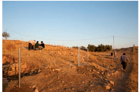
New fences, surrounding the excavation areas were built as well (Photo: NB).
